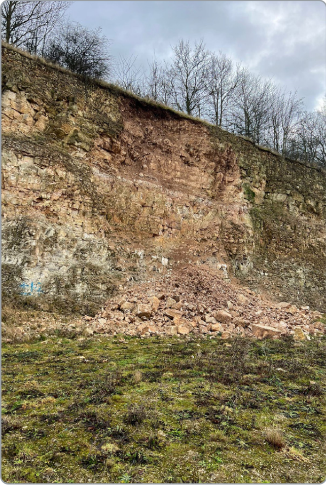
Localise face failure
