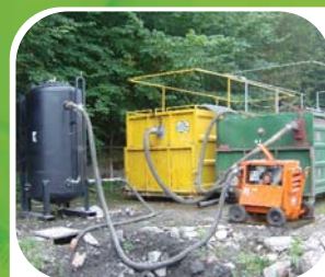
Mobile oil/water separator plant with final filtration to treat groundwater contaminated with hydrocarbons at a site in Aberdeen.
